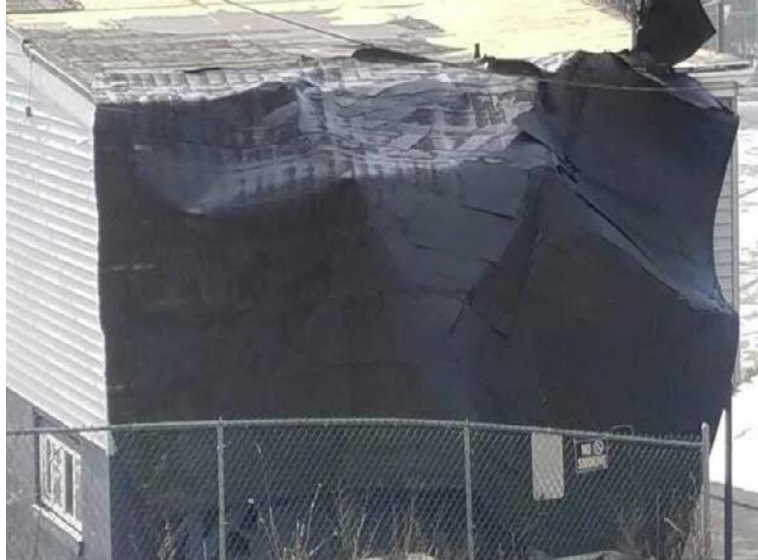
Figure 105: Damage to the Rensselaer Little League Field Concession Stand (CBS6 News)
