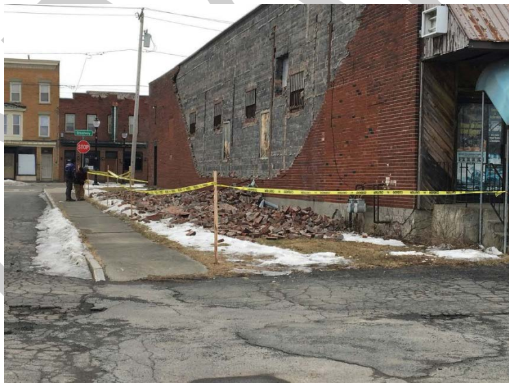
Figure 106: Damage to an Auto Parts Store in the City of Rensselaer (CBS6 News)
