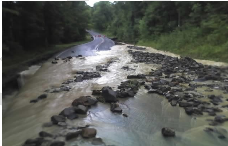
Figure 87: 1996 Flood Event -Road Washed Away in Rensselaer County
