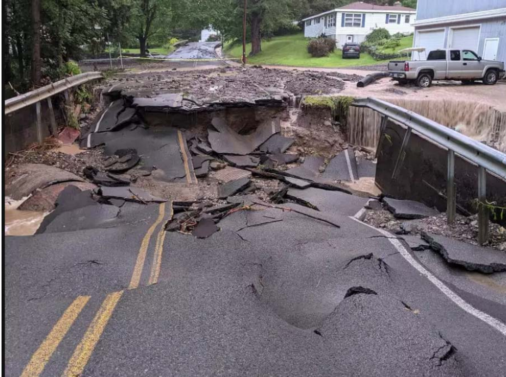
Figure 92: July 14, 2021, Heavy Downpours Damage Roads in Central and Southern Rensselaer County, Including This portion of Taborton Road in the Town of Sand Lake 93
